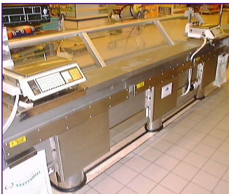
Three unit Fogging system
